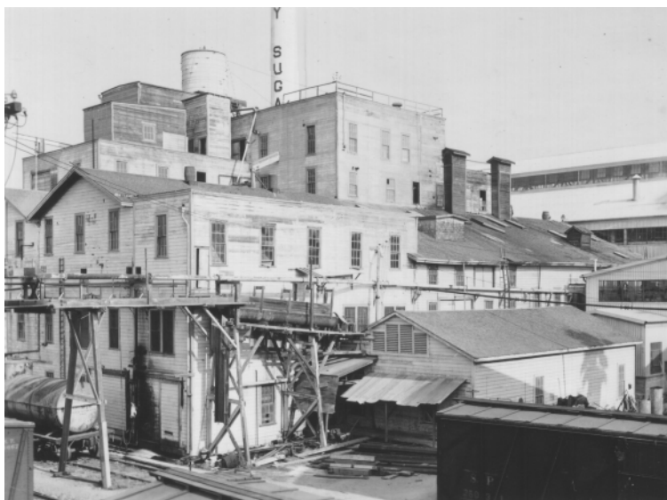
Old wooden factory being torn down as new metal factory is being built
